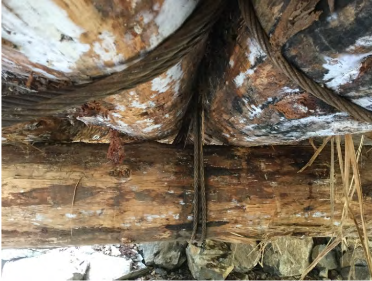
Needle beam not sufficiently tight to stringers
